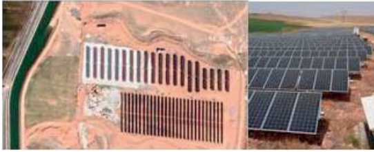
Figure 4. Single-axis tracking solar PV plant
