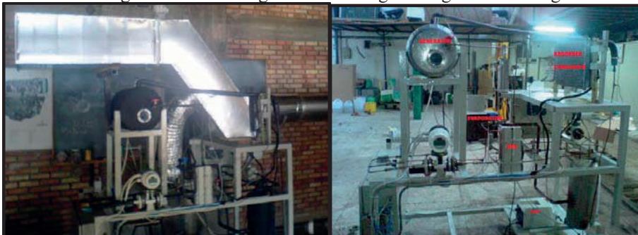
Figure 4. Experimental set-up of LiBr/Water Absorption Refrigeration System
